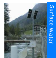
Station with Solar
